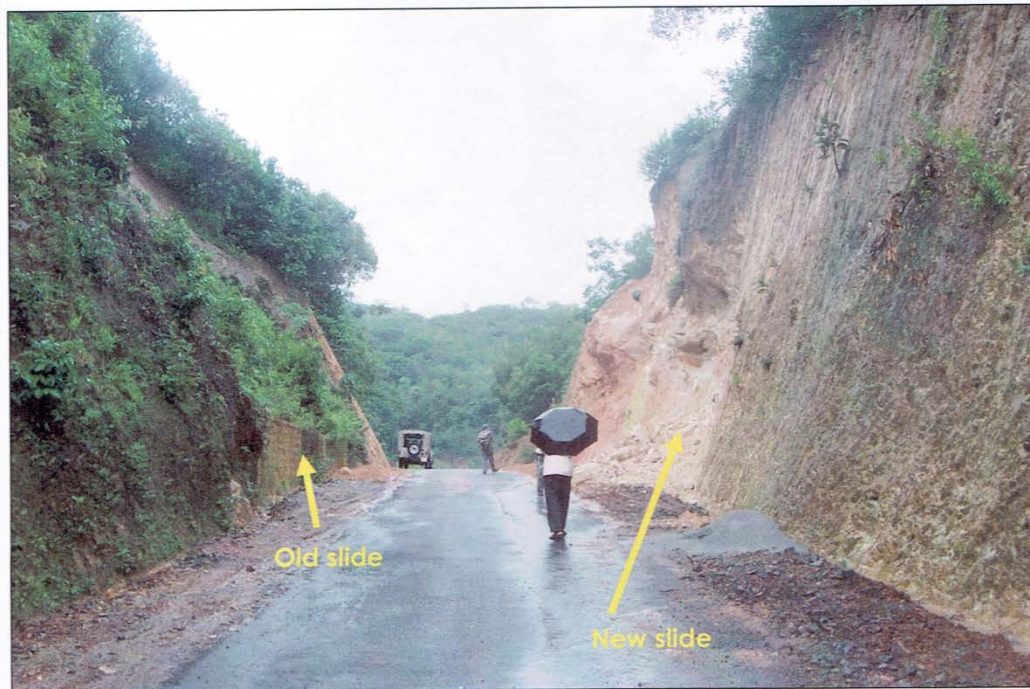
Photo 3: landslide near Onibagilu on Peruvai- Pakalkunja road connecting Vittla and Manila. The right side of the road is new slide and left side is the old stabilised slide.
