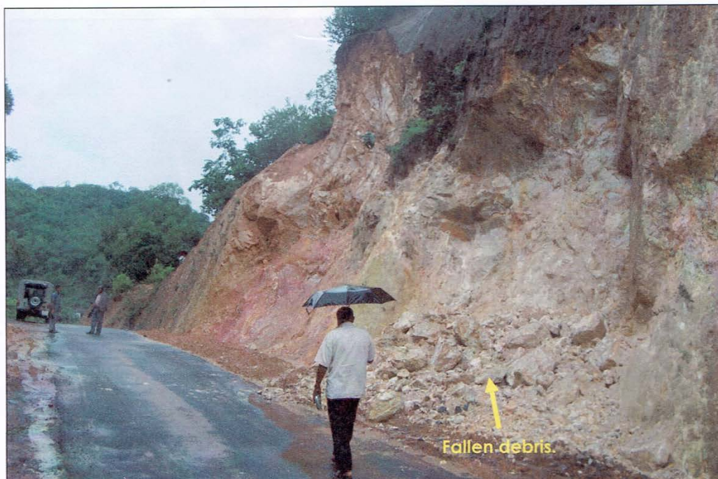
Photo 4: landslide near Onibagilu on Peruvai- Pakalkunja road connecting Vittla and Manila with fallen debris on toe part of the slide.
