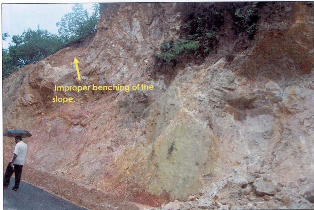
Photo 6: Improper benching at the mid slope, proper extension of bench to whole slope might have prevented the slide.
